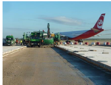
Düsseldorf Int. Airport, Reconstruction TWY L7 (© pictures, as no further mention: A.C.E. GmbH)
